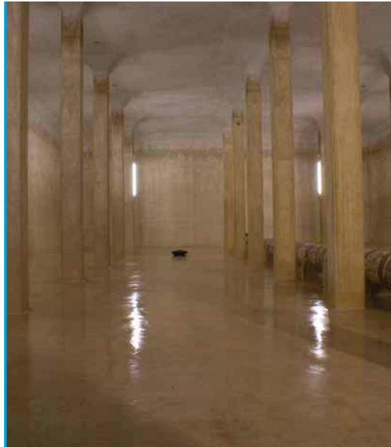
Underground drinking water reservoir
