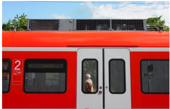
Air-conditioning system on a train roof.
